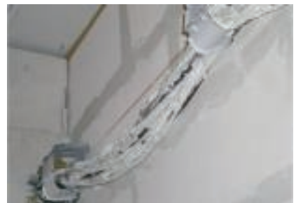
The copper conductors remain separate from one another – no short-circuit is created.
